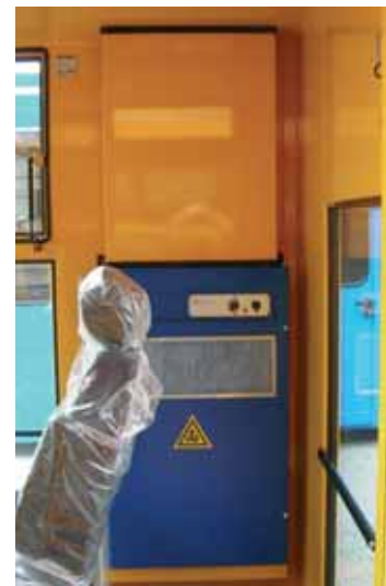
Air Conditioner inside view
