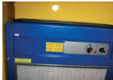
Air Conditioner control panel detail
